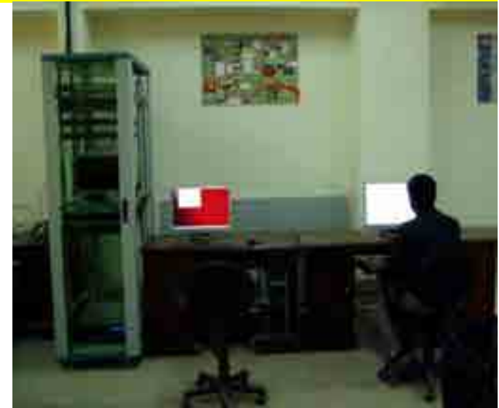
Central Data Collection Hub National Seismic Control Room
